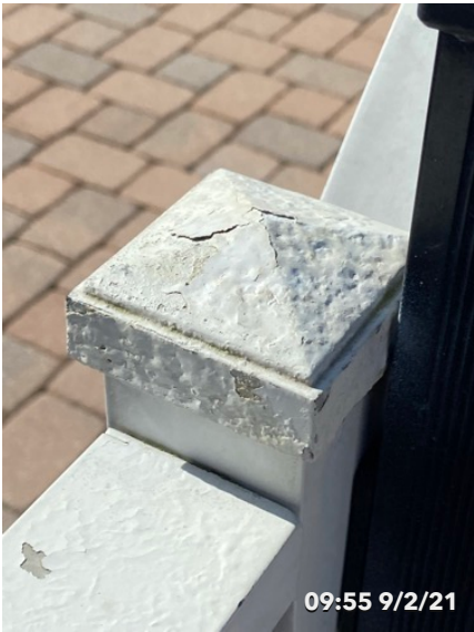
Observation 10 Refurbish gate to kiddie pool
