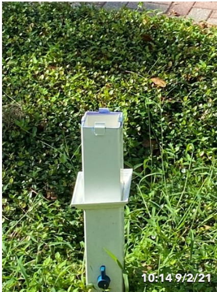
Observation 4 Replace cap water spigot unit at Town square.
