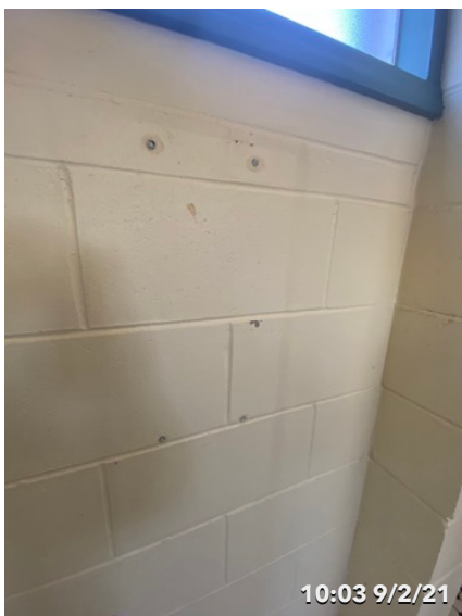
Observation 6 Remove wall plugs and caulk and paint in similar color at swim club bathroom
