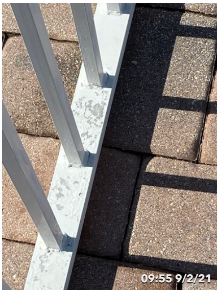
Observation 9 Refurbish and paint gate to kiddie pool.
