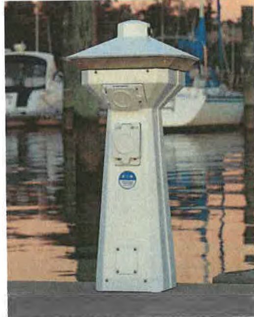
Hatteras Light Power Pedestal
