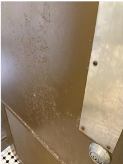
Observation 21 Sand and paint inside bathroom doors Swim club
