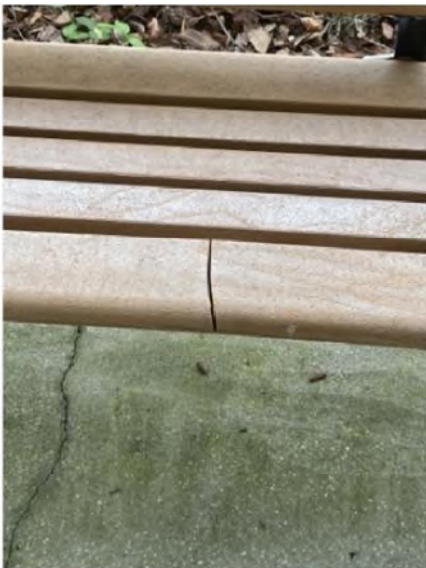
Observation 12 Crack in bench needs repair pocket park Primrose willow
