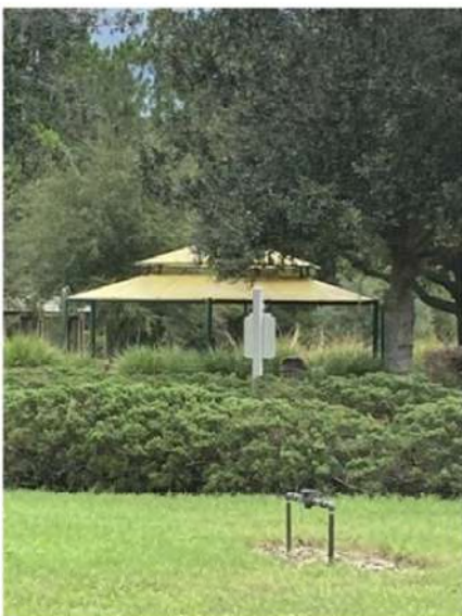
Observation 13 Pavilion roof need soft pressure wash
