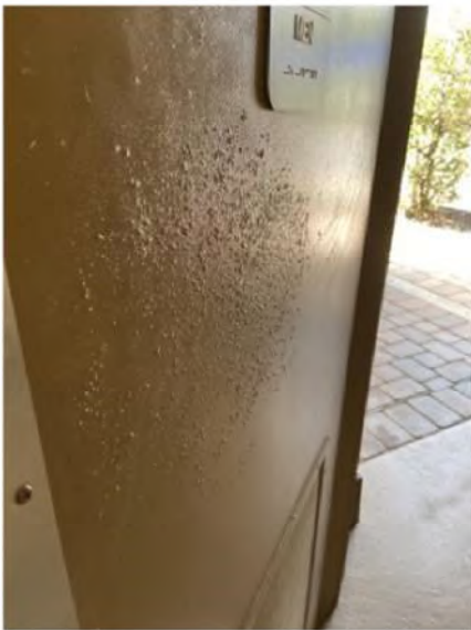
Observation 18 Sand and paint doors outside bathrooms Swim Club
