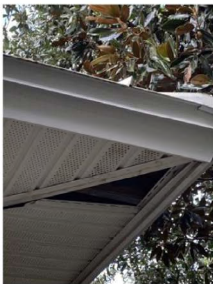
Observation 33 Repair soffet
