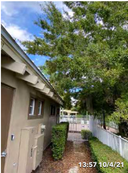
Observation 5 Servello Servello Tree trimming needed behind Swim Club
